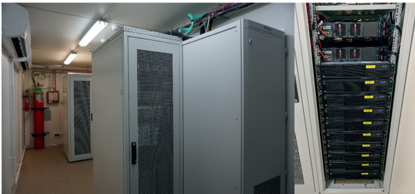
Figure 7 Mobile data processing centre installed in a 40 ft container.
